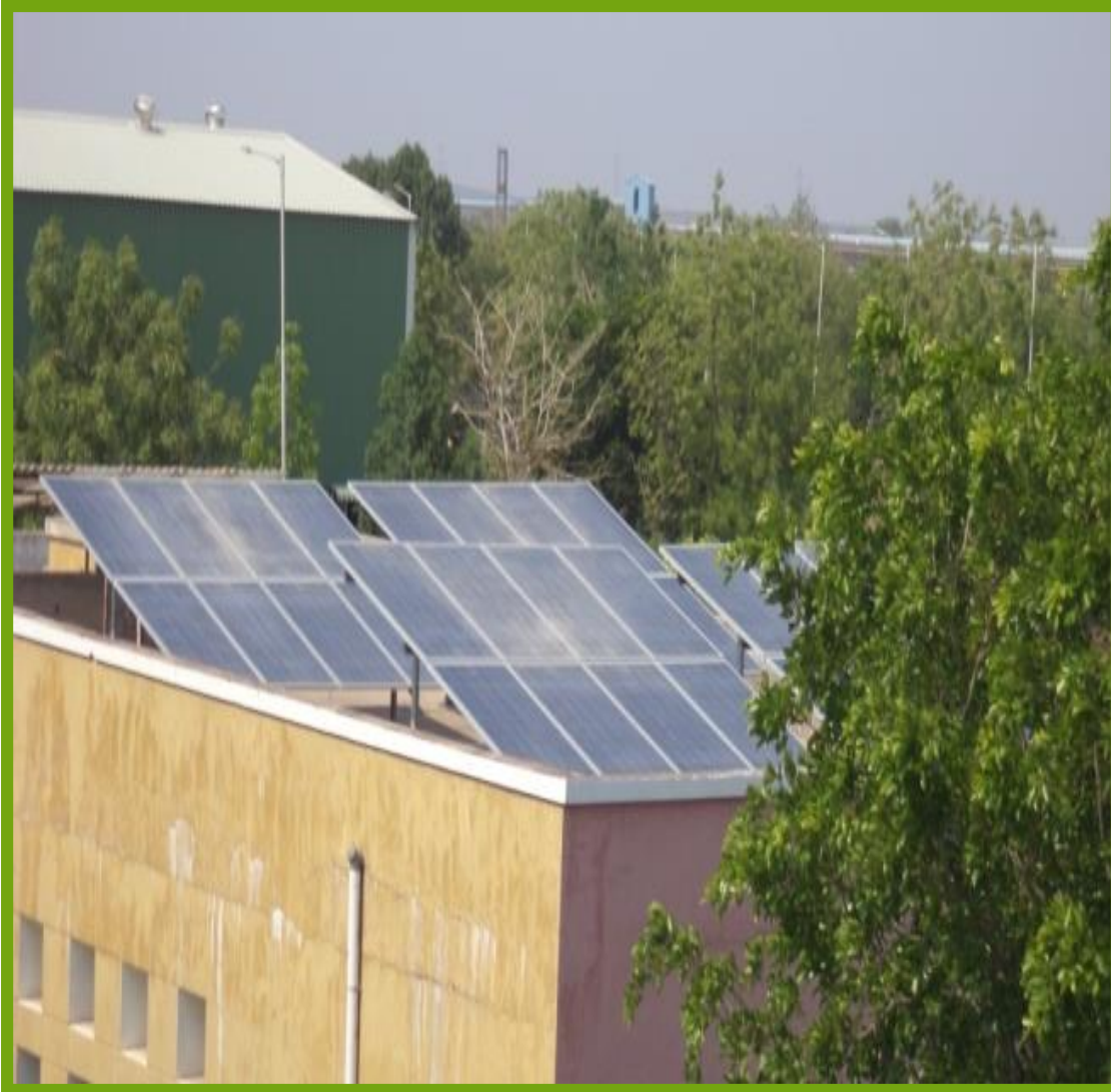
Solar Roof Top-30 KW at Guest House
