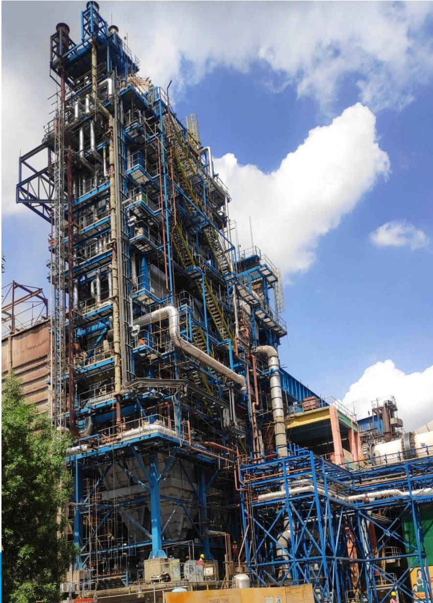
AQC Boiler – WHRS
