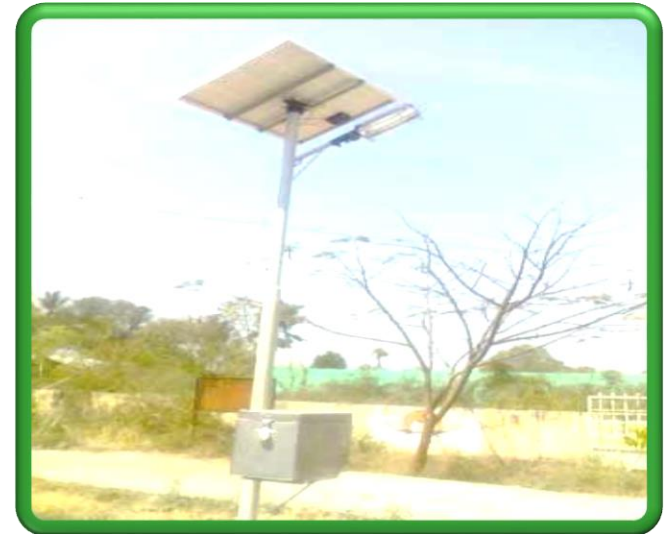
Solar Street Lights(8 Nos)
